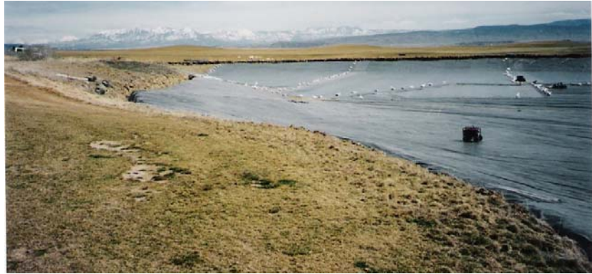
Installing a liner at the Devil's Thumb Golf Course pond (Photo: Delta County)
